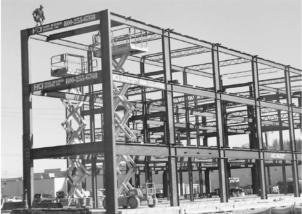
FIGURE 13.12 Multistory metal building system with moment-resisting rigid frames and open-web steel joists. ( HCI Building Systems, Inc. )
